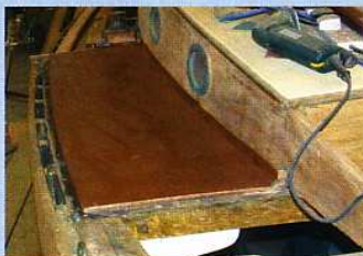
The cabin-to-deck joint may leak
